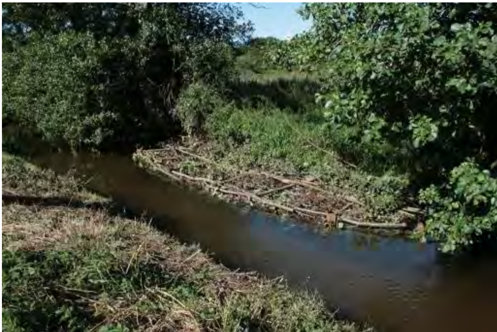
Photo 15 Brushwood mattress consisting of branches from tree coppicing staked and battened or wired down. The mattress accumulated fine sediment and vegetates, narrowing and deepening the channel.
