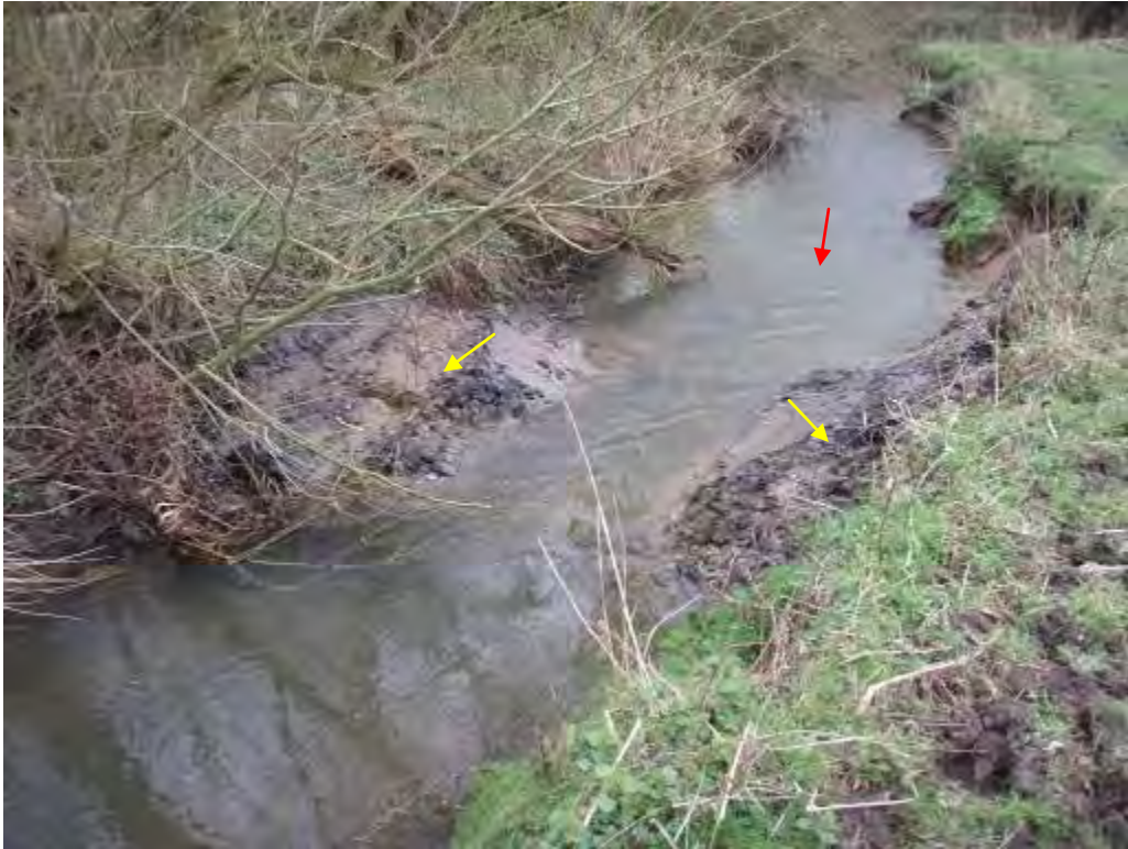
Photo 16 Direct remodelling of the river channel with an excavator can be a quick and cheap method of increasing the diversity of the channel form in lowland rivers. Here a deep pool has been excavated (red arrow) and the material used to make “shoulders” upstream of the pool (yellow arrows) to pinch the channel and create scour which will maintain the pool depth.
