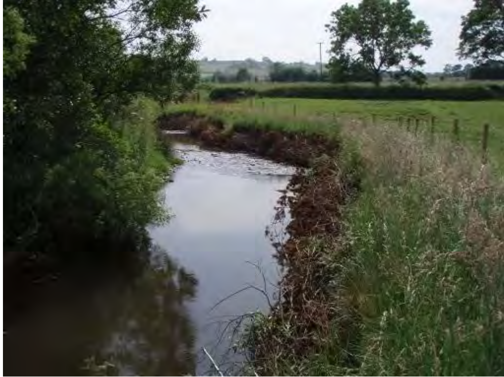
Photo 17 Brushwood revetment installed along an eroding bank, which was then fenced. Photo taken 8 months after installation. Trees have subsequently been planted here.
