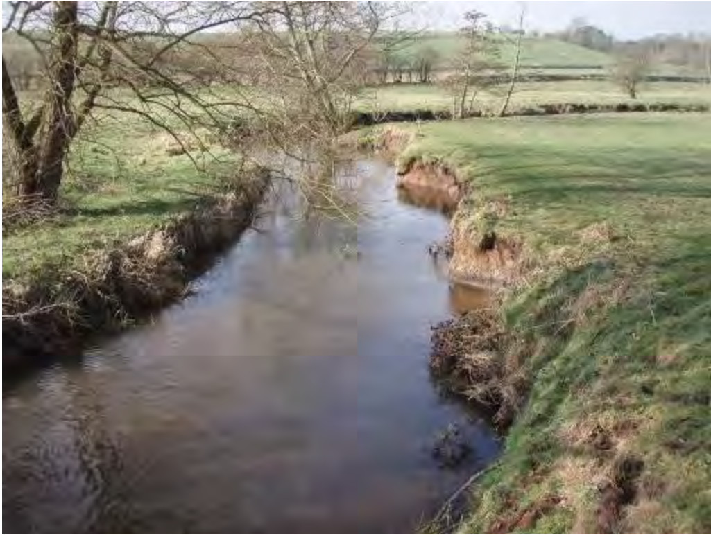
Photo 4 Areas with fewer trees tend to have accelerated rates of bank erosion and a wider, shallower channel. Bank revetment using “soft” techniques (brushwood) are necessary here along with buffer strip creation.
